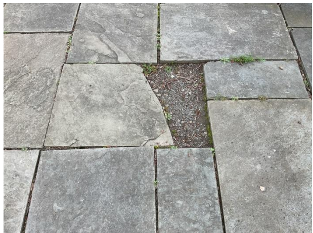
Broken bluestone paver
