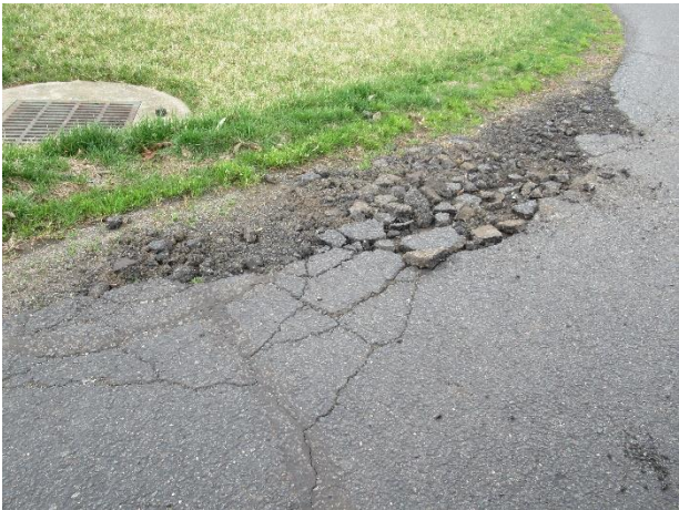
Edge deterioration and cracks at the alleys
