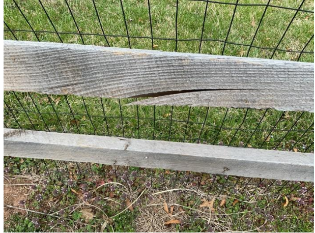
Wood split at split rail fence
