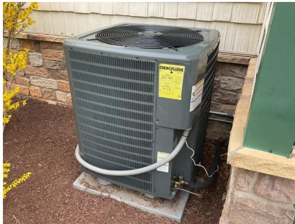
Condensing unit overview
