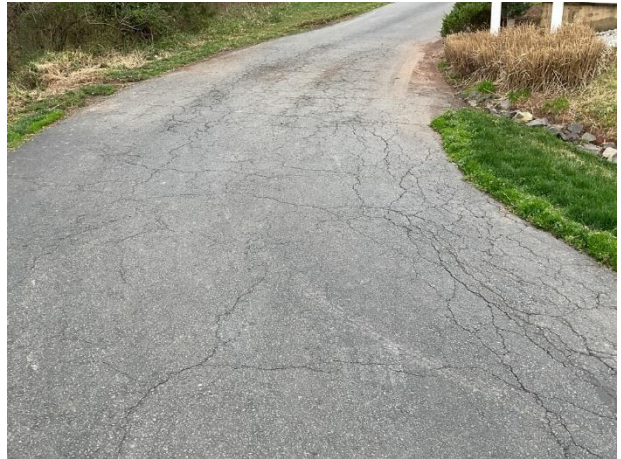
Cracks at alley
