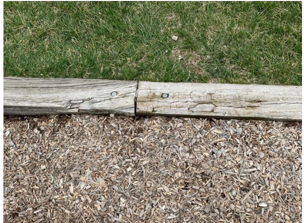
Wood border deterioration at Brown Thrasher Court playground
