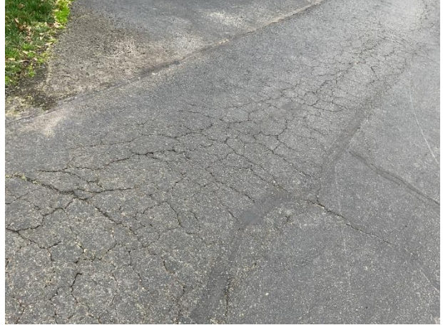
Cracks at alley
