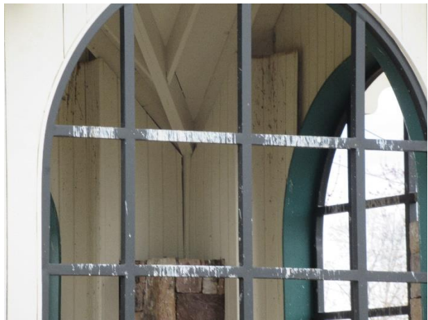
Stained metal railings
