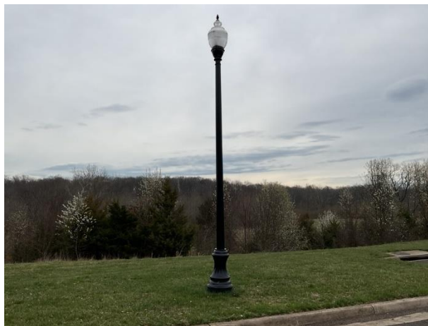
Light pole and fixture
