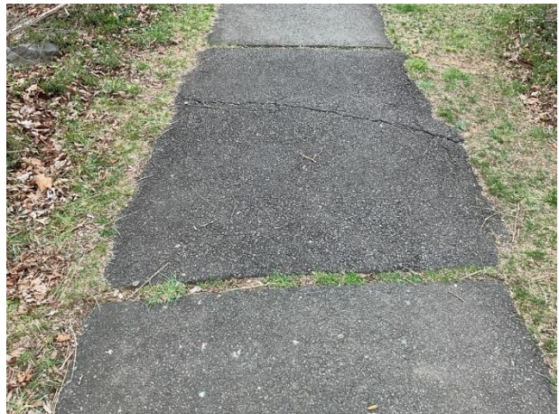
Pavement cracks and organic growth
