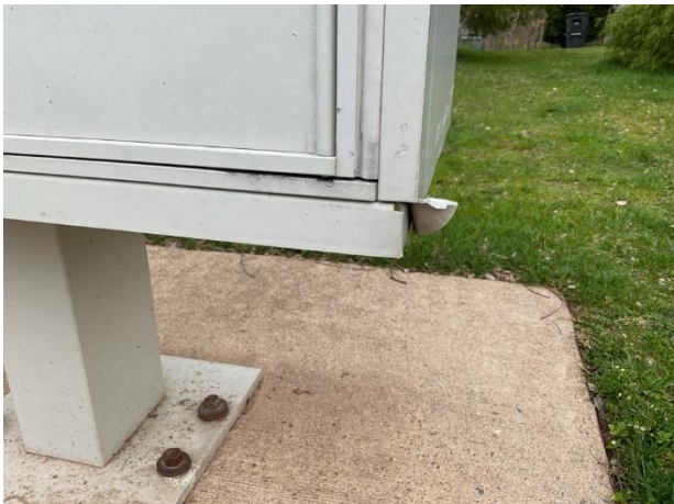
Damaged station at townhome mailboxes
