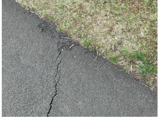
Pavement cracks and edge deterioration
