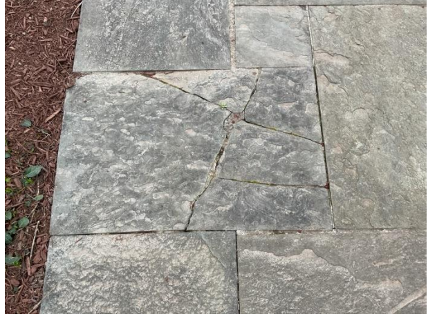
Cracked bluestone paver
