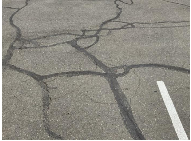
Cracks and prior repairs at the clubhouse parking area
