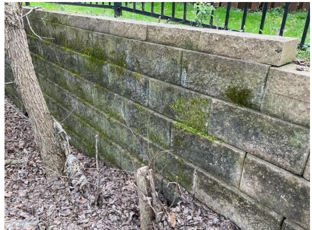
Organic growth at the masonry retaining walls
