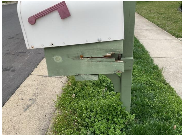
Wood rot at cluster mailboxes
