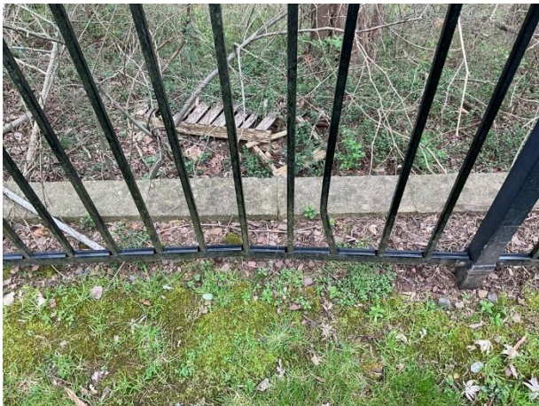
Damaged pickets and rail
