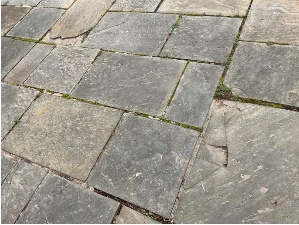
Cracked bluestone pavers
