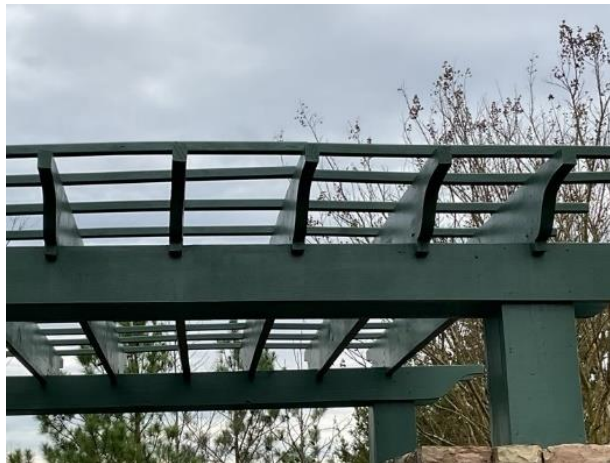
Warped boards at Yellow Hammer Drive
