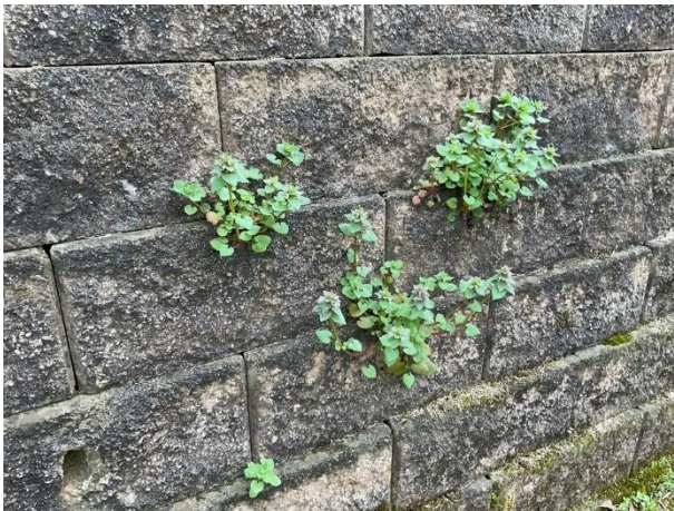
Organic growth at the masonry retaining walls
