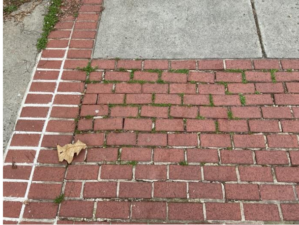
Mortar deterioration and organic growth
