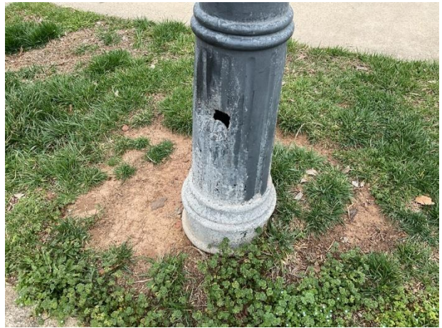
Damaged base and finish deterioration
