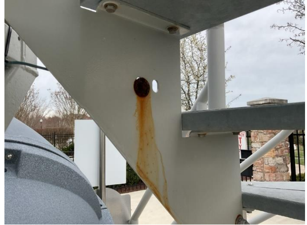
Fastener rust and rust stains
