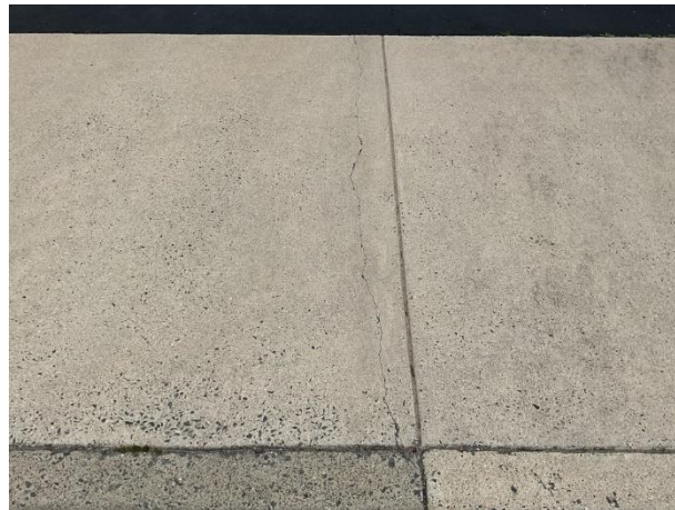
Concrete crack and scaling
