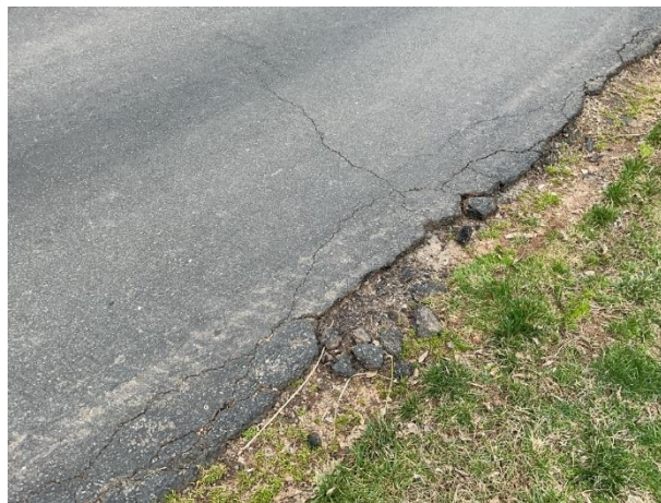
Edge deterioration and cracks at the alleys
