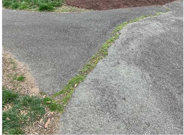
Pavement cracks and organic growth
