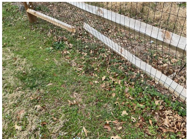
Broken rail at split rail fence
