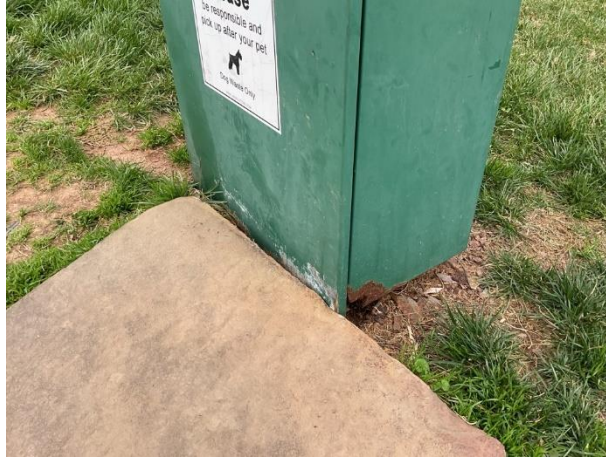
Finish deterioration and rust evident
