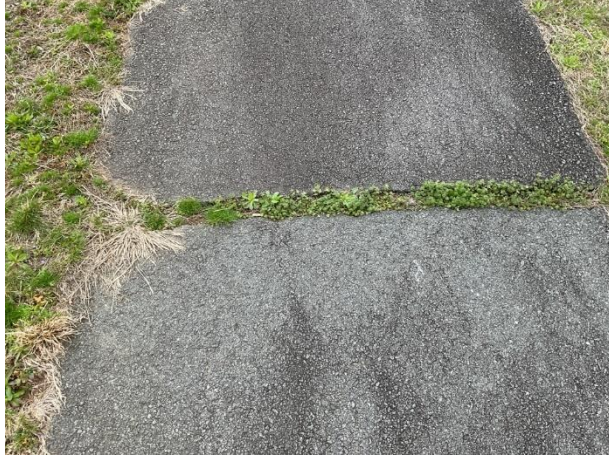
Pavement cracks and organic growth
