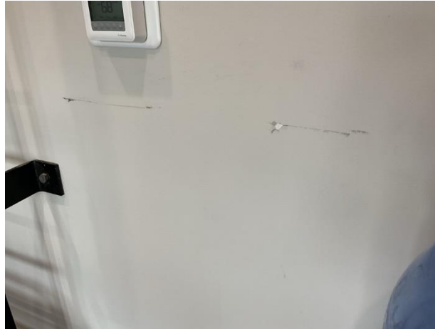
Paint finishes deterioration
