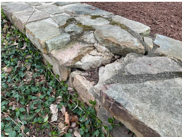
Missing stones at the stone retaining walls
