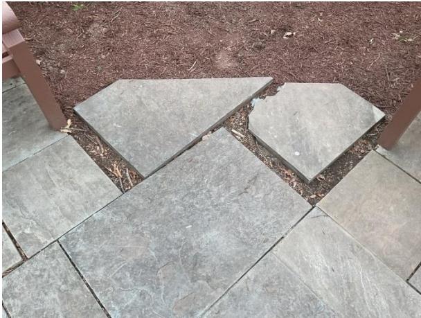
Displaced bluestone paver
