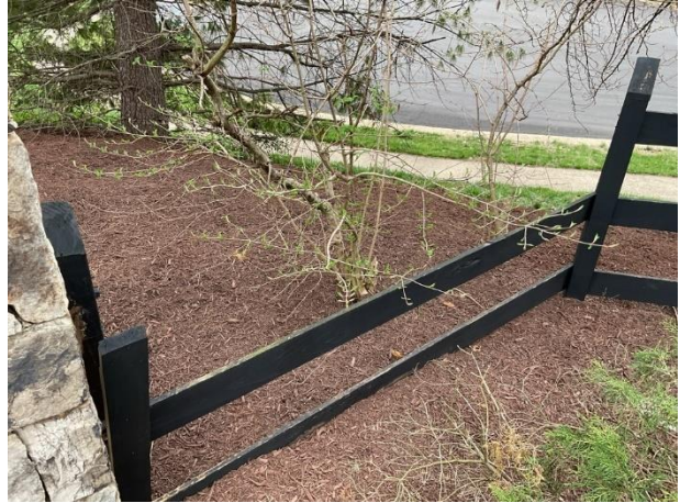
Missing and loose boards at open rail fence
