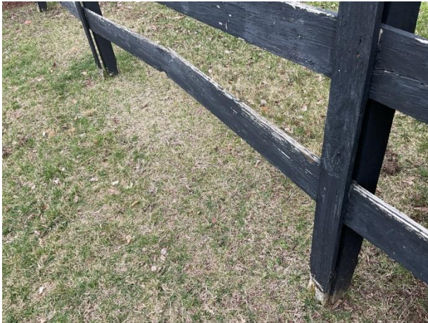
Damaged board and finish deterioration and open rail fence
