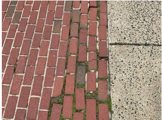
Mortar deterioration, masonry crack and organic growth at masonry pavers
