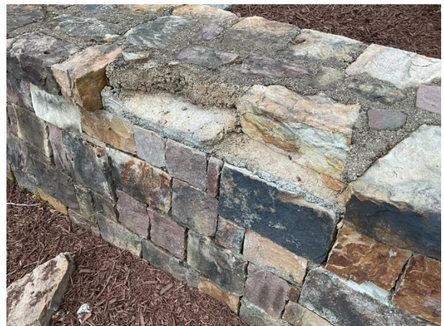
Missing stones at the stone retaining walls
