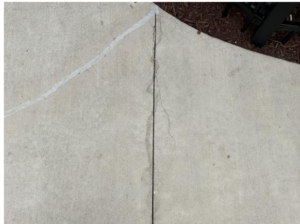
Concrete cracks and prior repairs
