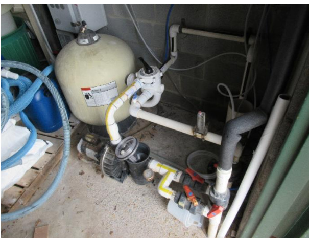
Wading pool pump and filter
