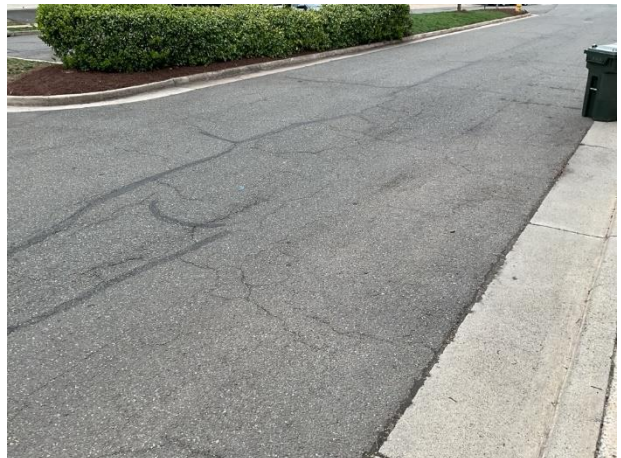
Cracks and prior repairs at the townhomes
