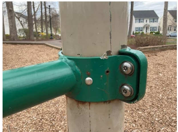
Finish deterioration at Parula Way playground
