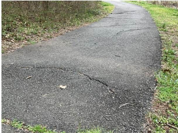
Pavement cracks and heaving due to root intrusion
