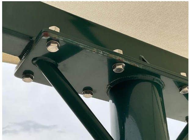
Finish deterioration and rust
