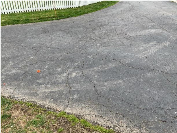
Cracks at alley
