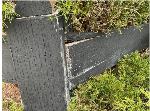
Wood split and finish deterioration at open rail fence
