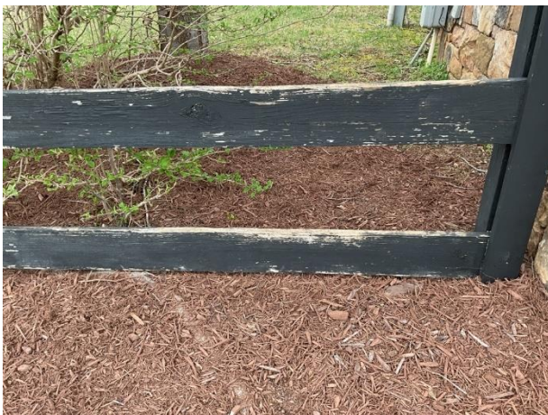
Finish deterioration at open rail fence
