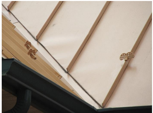
Warped roof overview
