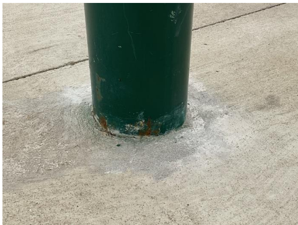
Finish deterioration and rust
