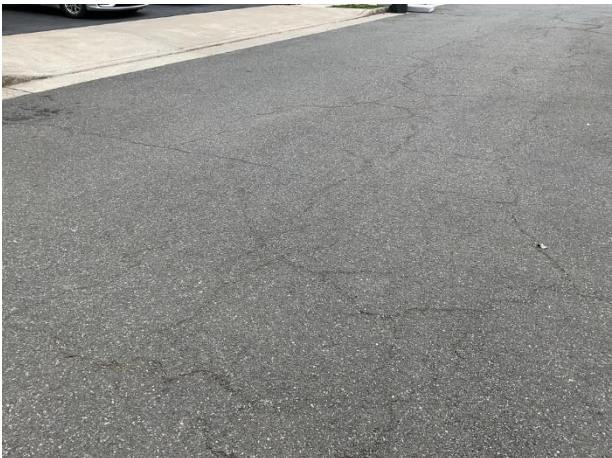
Cracks at townhome streets
