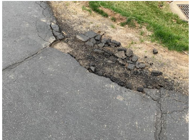
Edge deterioration and cracks at the alleys
