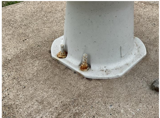
Fastener rust at townhome mailboxes
