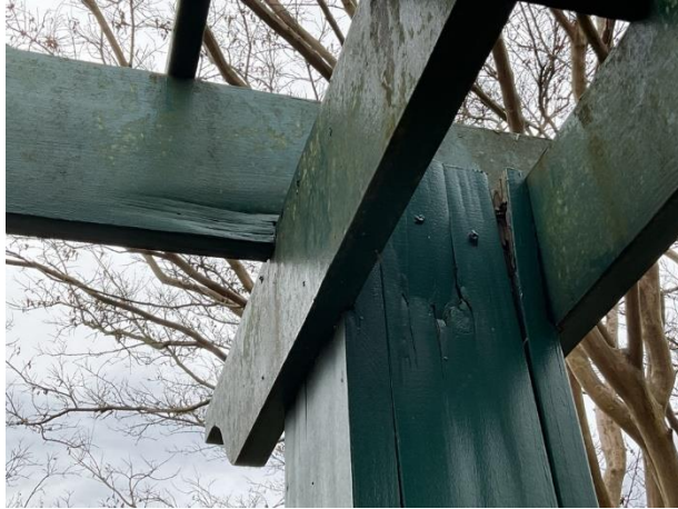
Wood deterioration at clubhouse
