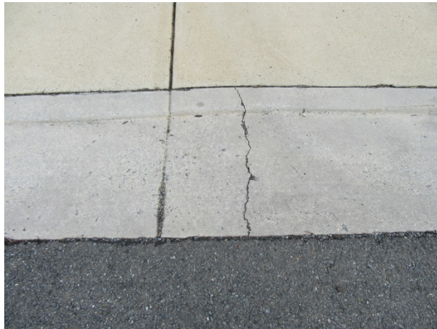
Curb and gutter crack
