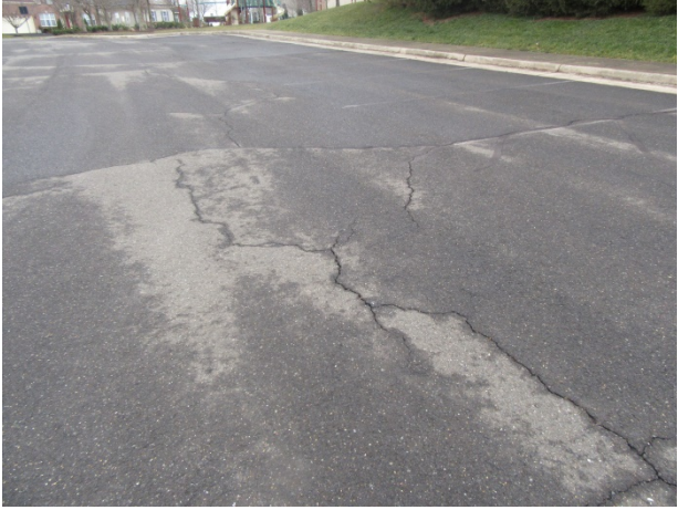
Cracks at the clubhouse parking area
