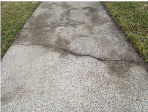
Sidewalk cracks and spall
