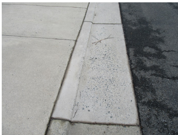
Curb and gutter spall
