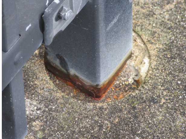
Steel fence rust
