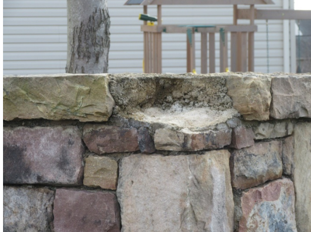
Missing masonry block at the entrance monument
