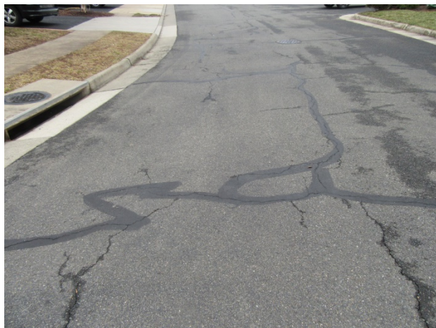
Pavement cracks and previous repairs at townhome pavement
