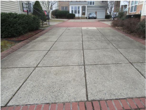
Driveway overview; we note concrete spall
