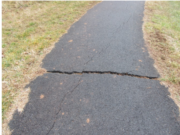
Walking path cracks
