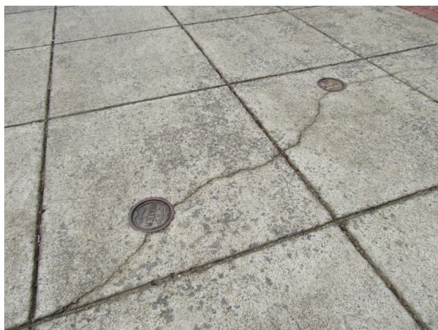
Concrete spall and cracks
