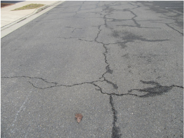
Cracks at townhome pavement
