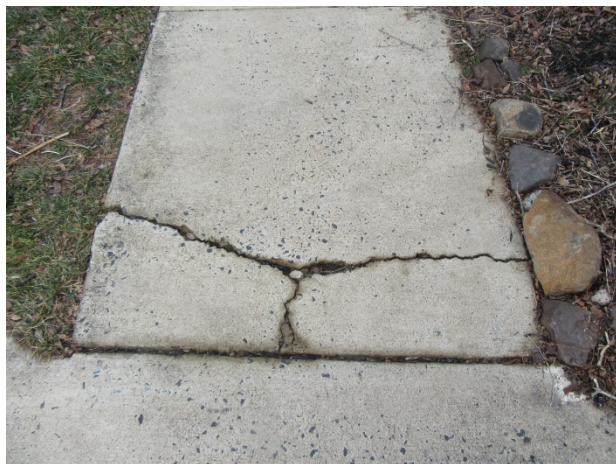
Sidewalk cracks, spall, and deterioration
