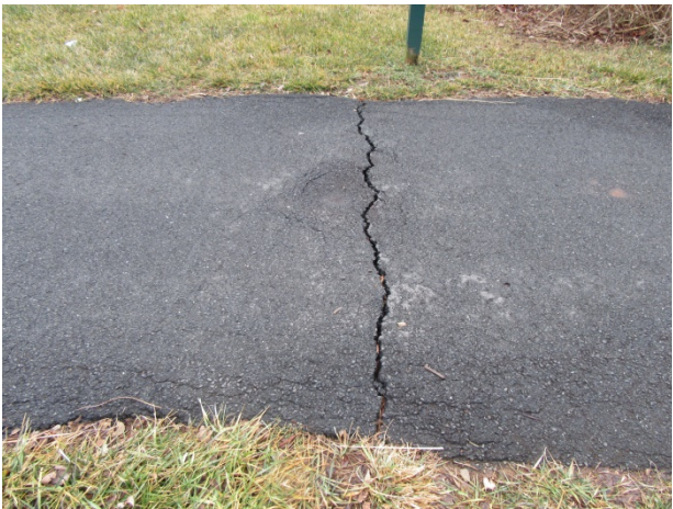
Walking path crack and settlement
