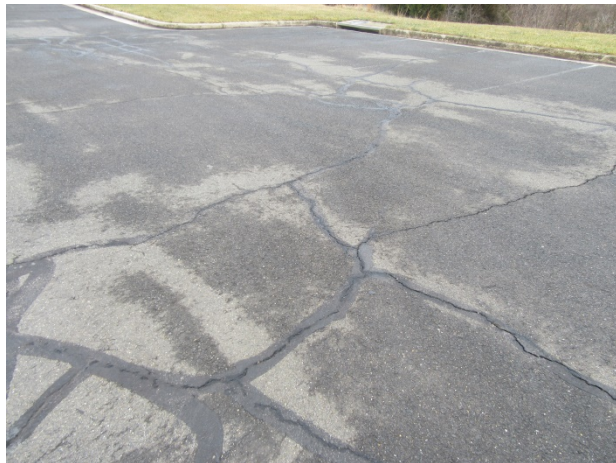
Cracks and previous repairs at the clubhouse parking area
