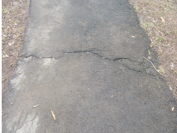
Walking path cracks
