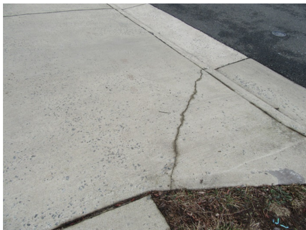
Apron crack and spall
