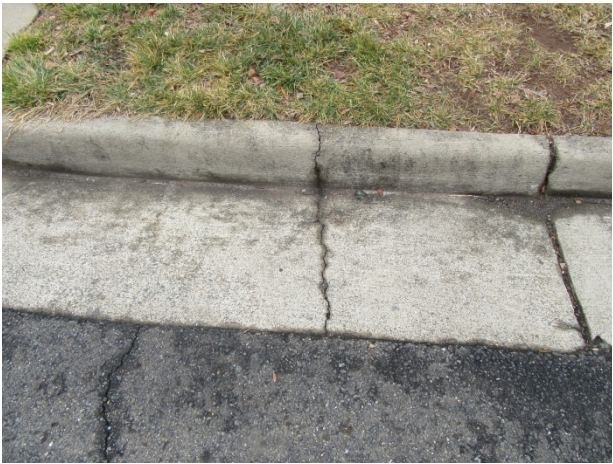
Curb and gutter crack
