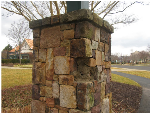
Missing stone veneer at the pergola masonry column
