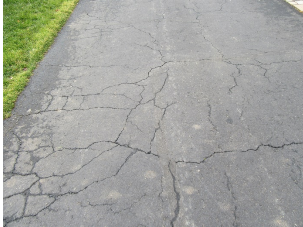
Cracks at Alley near Willet Way
