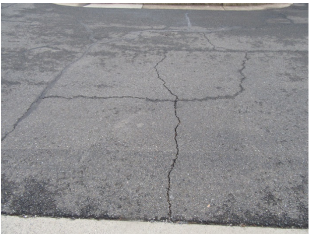
Pavement cracks at townhome pavement
