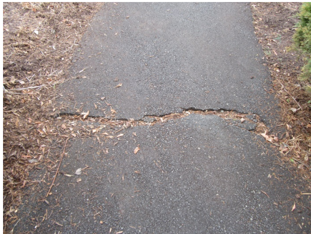
Walking path cracks
