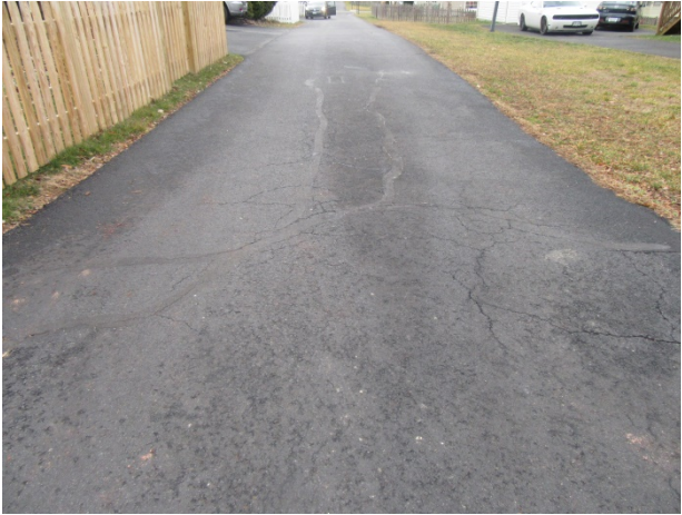
Alley; we note cracks and previous repairs
