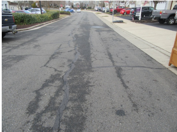
Previous repairs and cracks at townhome pavement
