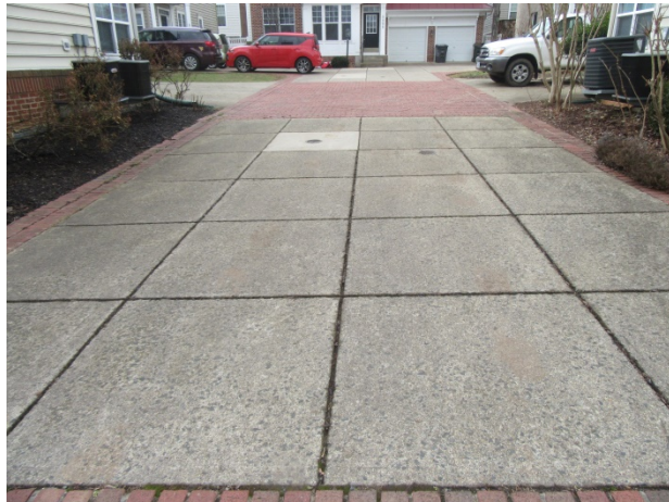
Driveway overview; we note spall
