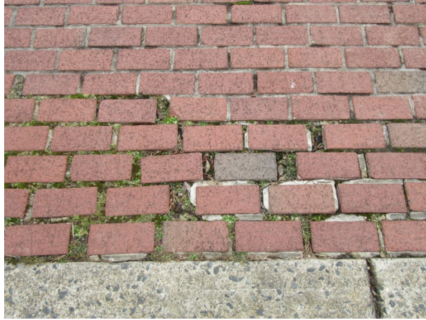
Pavers mortar deterioration
