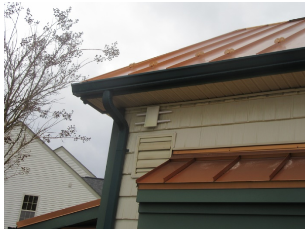
Aluminum gutter and downspout assembly
