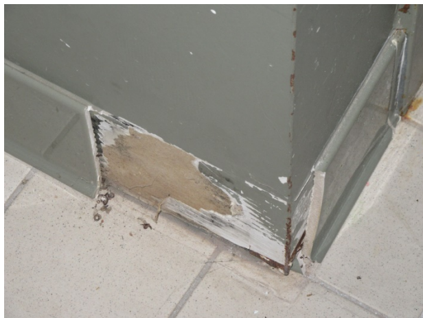
Clubhouse interior finish deterioration
