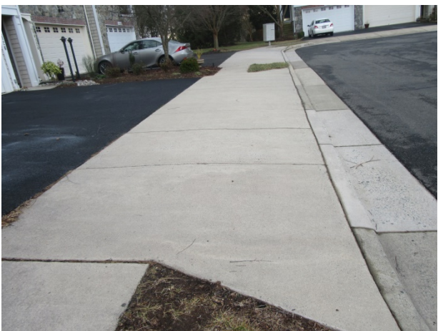
Concrete apron; we note spall
