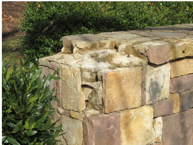
Missing masonry block at the arbor masonry wall
