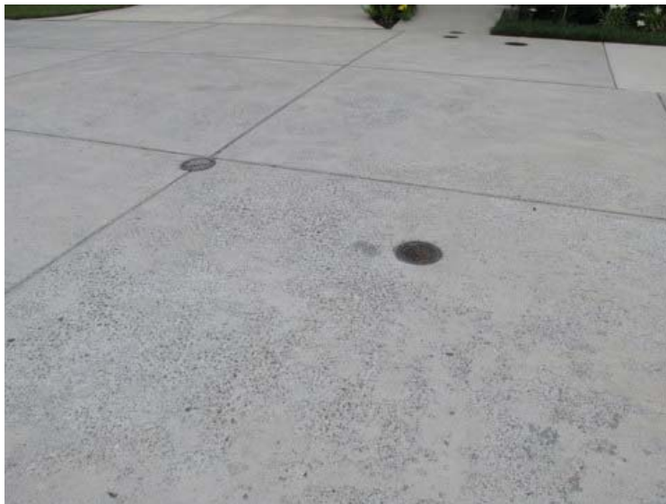
Concrete driveway spalls
