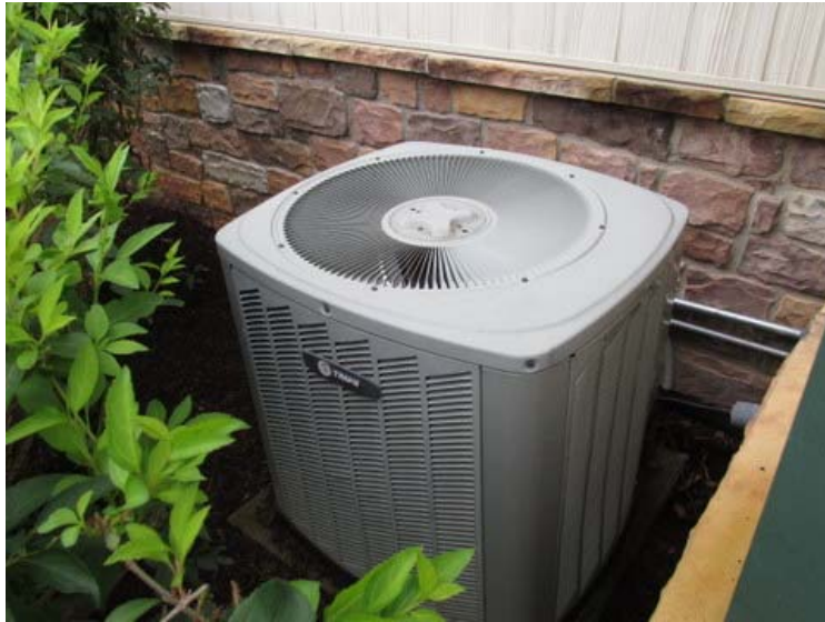
Clubhouse HVAC equipment
