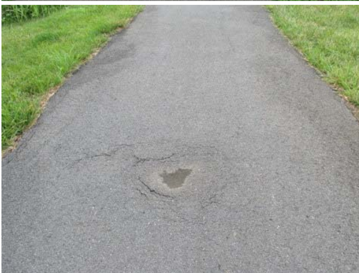
Pavement settlement at walking path
