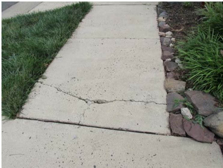
Cracked concrete sidewalk
