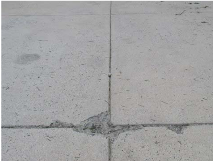
Concrete driveway deterioration
