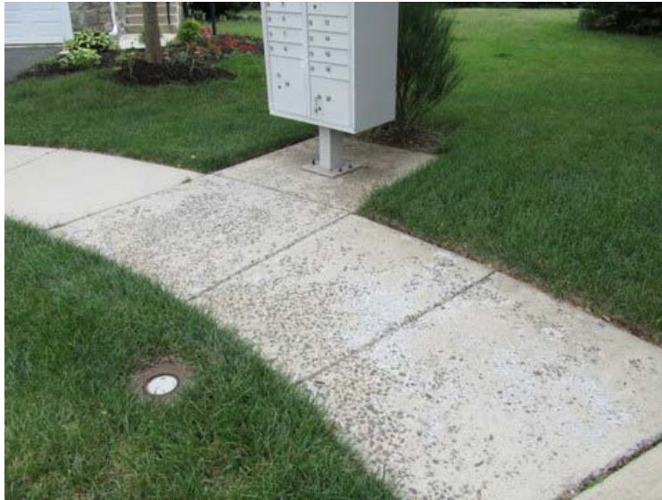
Concrete sidewalk spalls
