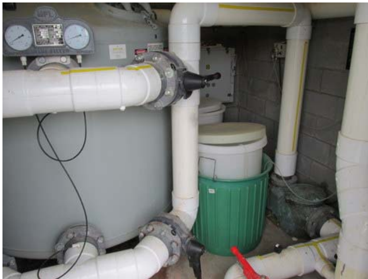
Pool filter and chemical storage
