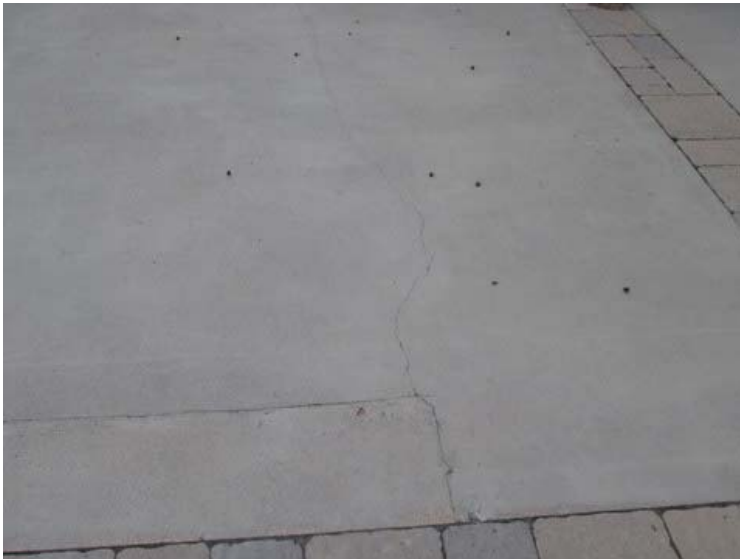
Cracks in pool deck
