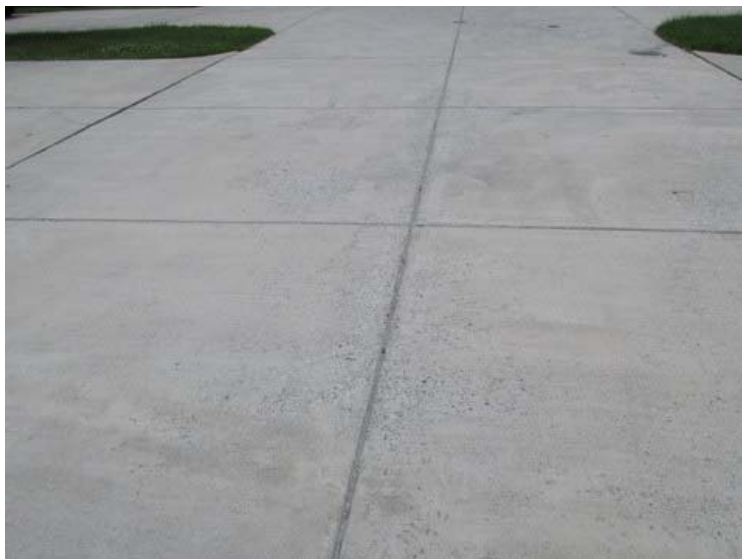
Concrete driveway spalls
