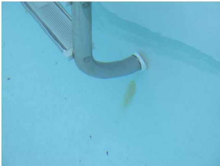
Rust stain at plaster finish
