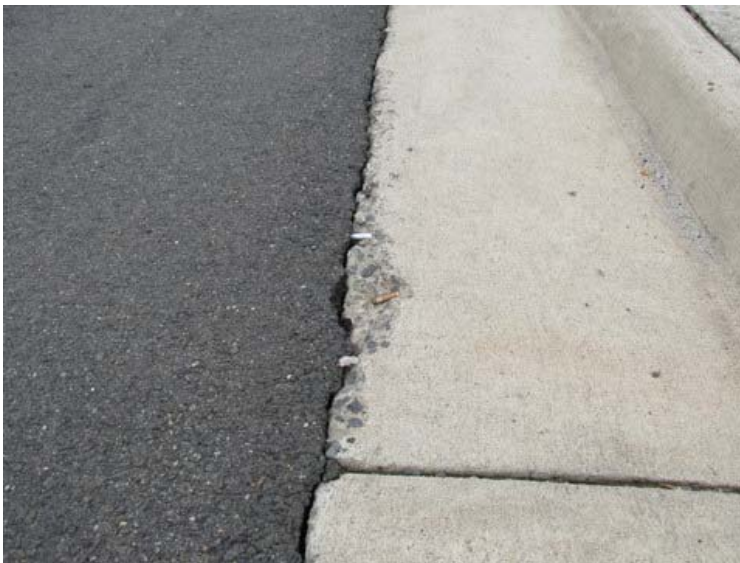
Damaged concrete gutter
