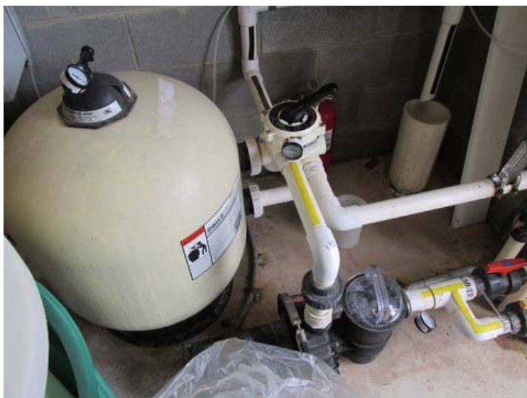
Filter and pump
