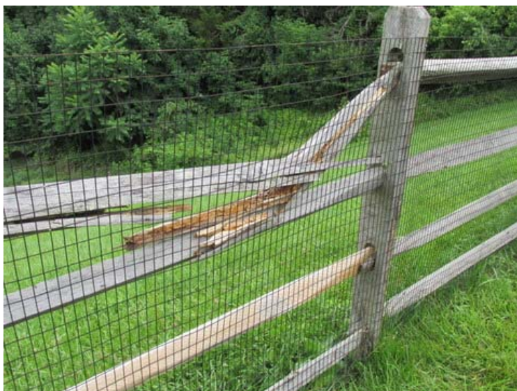
Damaged split rail fence atop earthen dam
