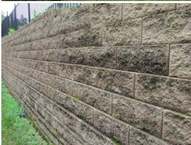
Water stains at masonry retaining wall
