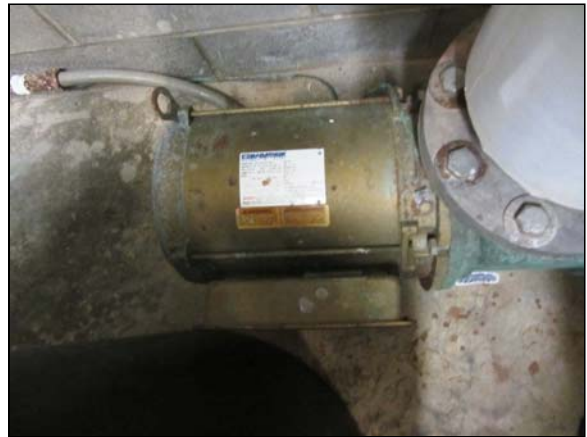
Photo #34. Main pool pump.
