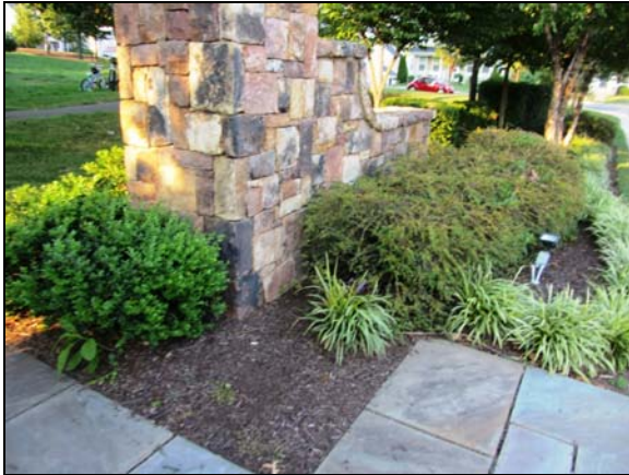
Photo #103. South entrance to Peacock Park. Note damaged ground mounted light fixture.
