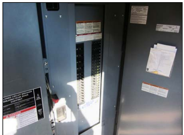
Photo #48. Electric service is located in a separate room on the west side of the Community Center.
