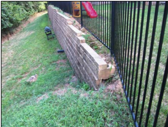
Photo #87. Typical erosion at the end of segmental retaining wall installations.
