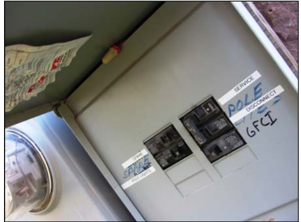
Photo #112. Electrical service at the Peacock Park Tot Lot indicates that the pole lights are the responsibility of the Association. Note wire nut above breakers.
