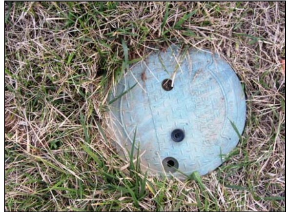
Photo #14. Underground vault for sprinkler equipment, Rollins Ford and Yellow Hammer.
