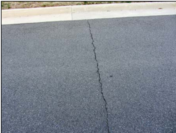
Photo #75. Open crack in the asphalt pavement.
