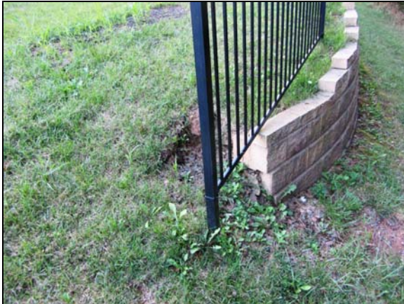
Photo #85. Typical erosion at the end of segmental retaining wall installations.
