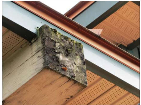
Photo #28. Deteriorated support beam at the Community Center.
