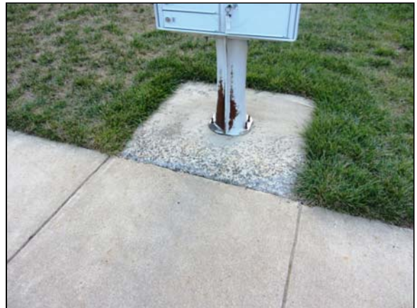
Photo #76. Deteriorated concrete pavement and deteriorated finish on the mailbox support post.
