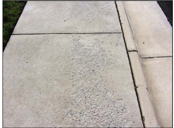
Photo #26. Typical deterioration of the concrete pavement near the swimming pool.
