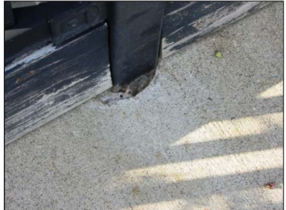
Photo #44. Fence posts are not properly installed into the concrete pool deck.
