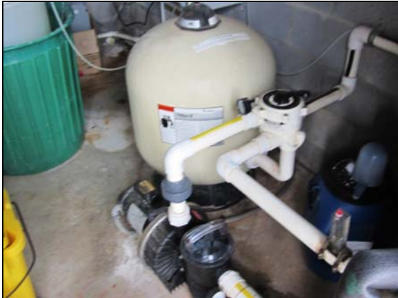
Photo #31. Wading pool pump and filter.
