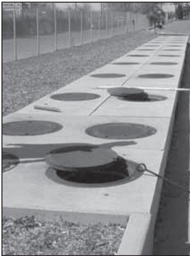
From the surface, some sand filters look like a series of manholes.
