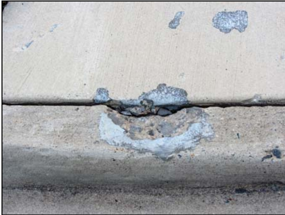
Photo #91. Concrete pavement and curb & gutter were repaired by patching and coating and they repairs have already failed.
