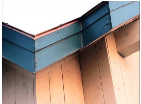
Photo #10. Failed paint system, Rollins Ford and Yellow Hammer.
