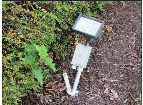
Photo #104. Damaged ground mounted light fixture at the south entrance to Peacock Park.
