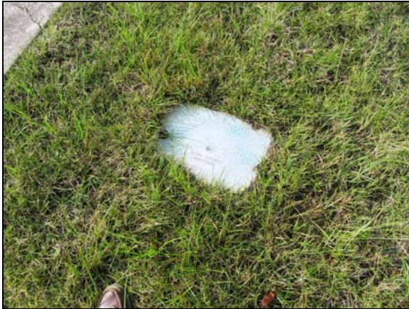
Photo #25. Underground vault for sprinkler equipment near the swimming pool.
