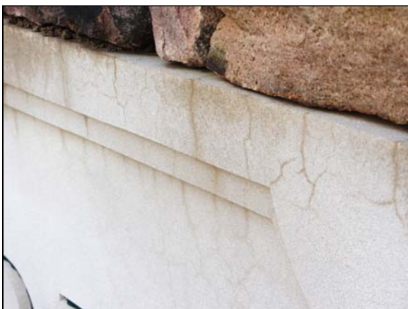
Photo #11. Hairline cracking of the precast property identification signage, Rollins Ford and Yellow Hammer.
