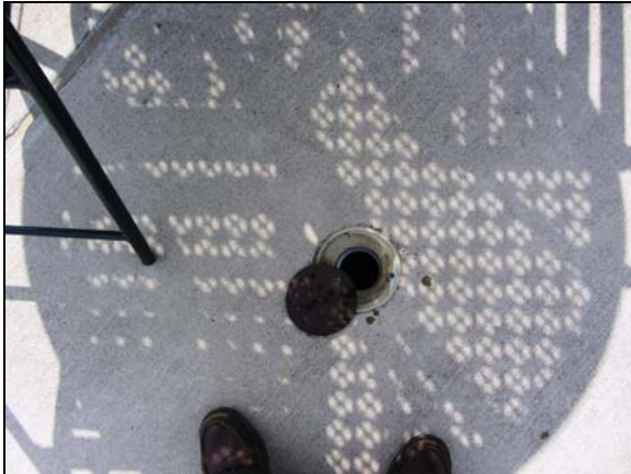
Photo #43. Loose drain cover near the wading pool is a potential trip hazard.
