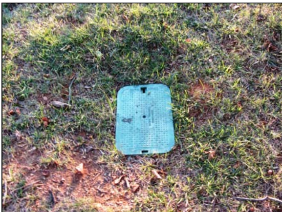
Photo #113. Irrigation vault at Peacock Park.
