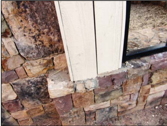
Photo #7. Rusty wire has been used to secure the precast simulated stone.
