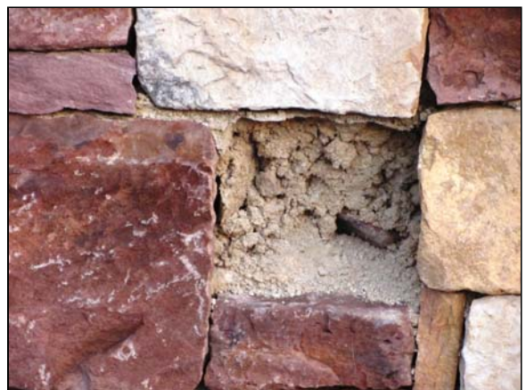
Photo #12. Typical missing precast simulated stone, Rollins Ford and Yellow Hammer.
