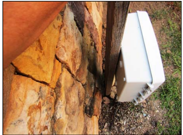
Photo #4. Irrigation controller is not properly mounted, Rollins Ford and Yellow Hammer entrance.
