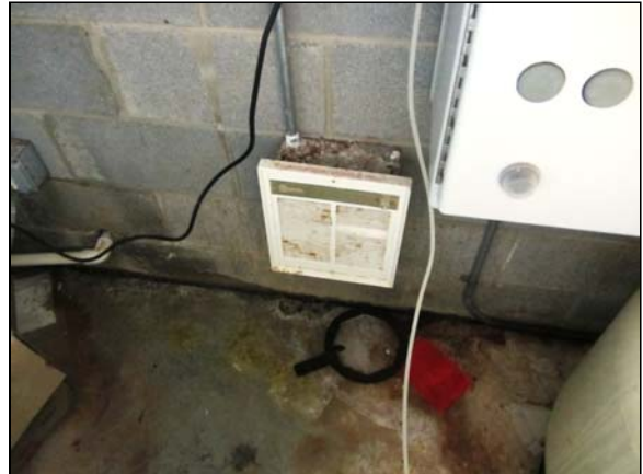
Photo #32. Small electric heater in the wading pool pump room.
