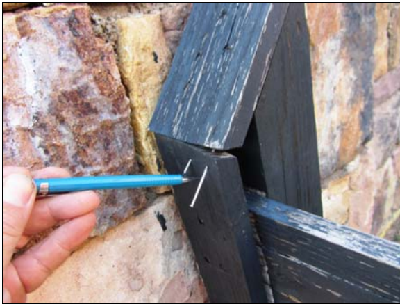
Photo #3. Minor defects in the wood fence at the Rollins Ford and Yellow Hammer entrance.
