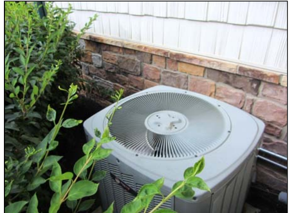
Photo #50. Community Center compressor.
