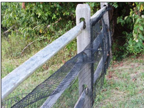
Photo #83. Minor damage to the metal fence attached to the rail fencing surrounding the dry pond.
