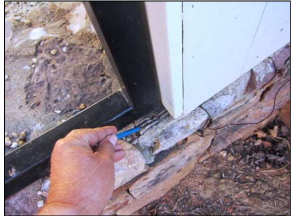
Photo #8. Deteriorated plywood extends from the upper surface of the structure.
