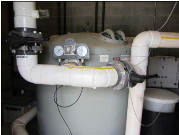
Photo #33. Main pool filter.
