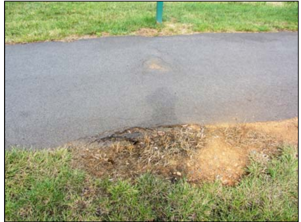
Photo #20. Defective grading adjacent to the asphalt trail and deteriorated asphalt trail east of the swimming pool.
