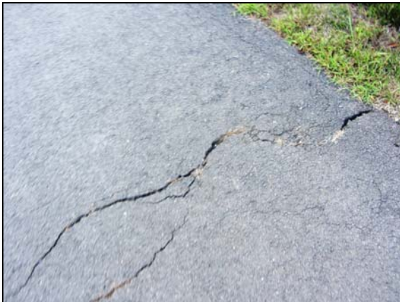
Photo #81. Typical crack in the asphalt trail.
