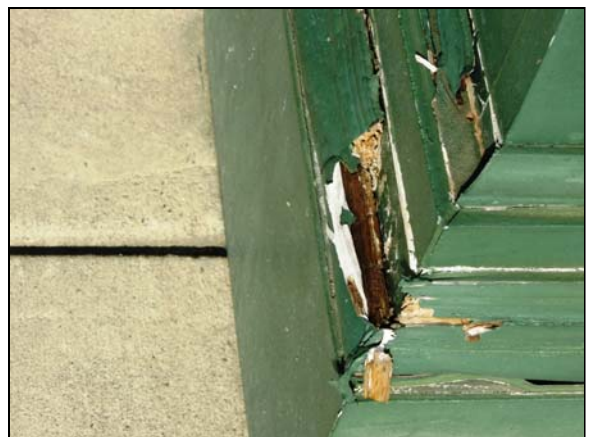
Photo #42. Deteriorated wood components of the pool deck trellis.
