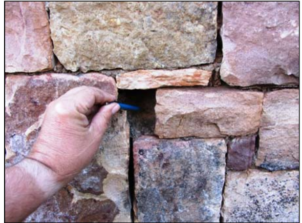
Photo #2. Missing precast simulated stone.
