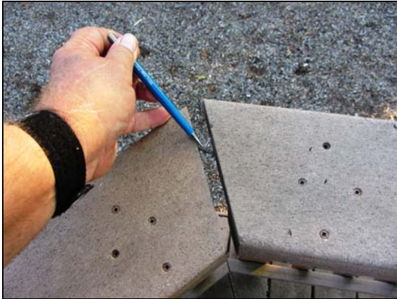
Photo #111. Defective deck railing in the Peacock Park Tot Lot area.
