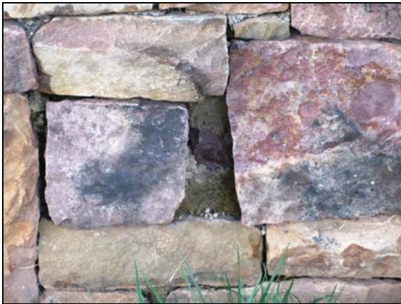
Photo #9. Typical missing precast simulated stone, Rollins Ford and Yellow Hammer.
