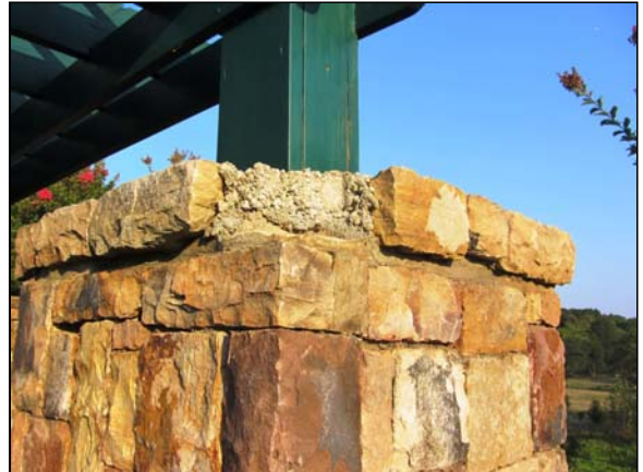
Photo #98. Typical defective precast simulated stone veneer at the sitting area south of Yellow Hammer.
