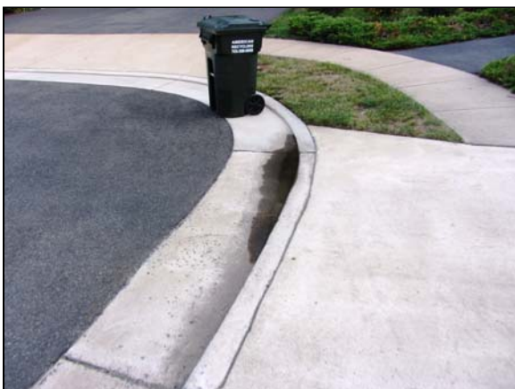
Photo #77. Concrete curb is not properly pitched to move water to the storm water system.
