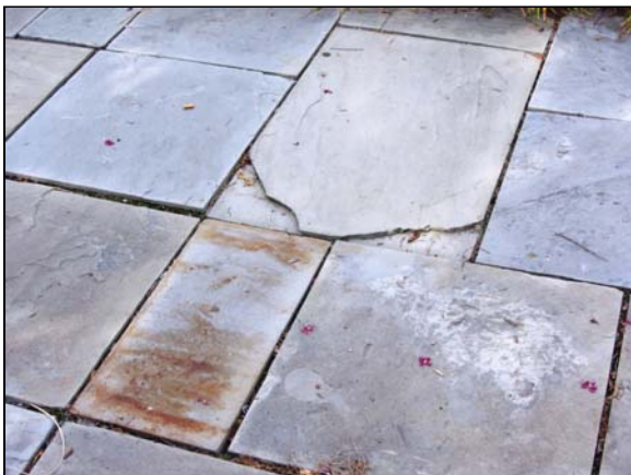
Photo #23. Deteriorated flagstone paver at the sitting area east of the swimming pool is a potential trip hazard.
