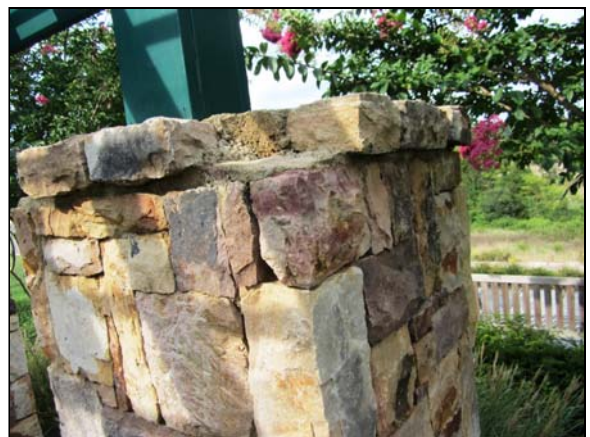
Photo #18. Typical missing precast simulated stone at the post supporting the trellis at the sitting area east of the swimming pool.
