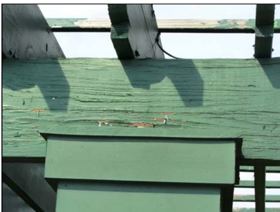
Photo #41. Failed paint system on the pool deck trellis.
