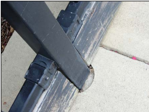
Photo #45. Fence posts are not properly installed into the concrete pool deck.
