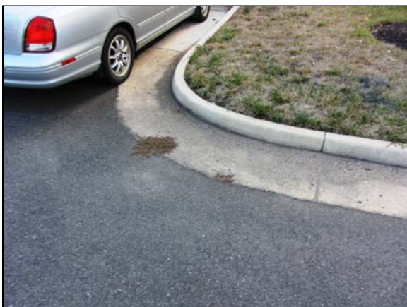
Photo #89. Asphalt pavement and concrete curb & gutter are not properly pitched to move water to the stormwater system.
