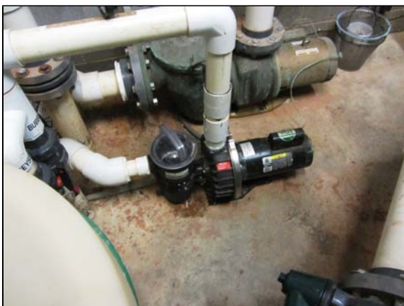
Photo #35. Pumps that serve the main pool umbrella and bubbler features.
