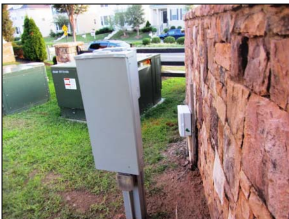
Photo #5. Electrical service at the Rollins Ford and Yellow Hammer entrance
