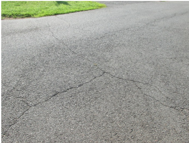
Pavement cracks at alley
