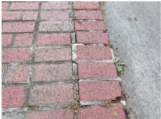
Mortar deterioration at pavers
