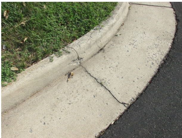
Curb and gutter crack
