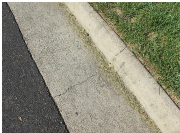
Curb and gutter crack
