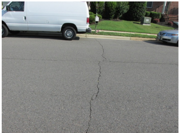
Pavement cracks at townhome pavement
