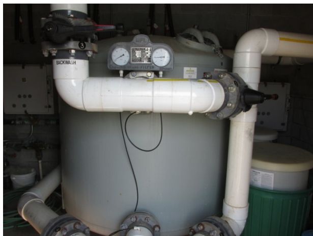
Main pool filter
