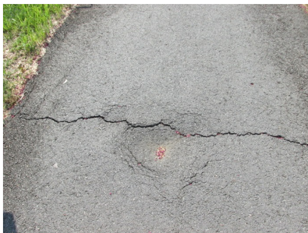
Walking path cracks and settlement
