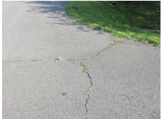
Pavement cracks at alley
