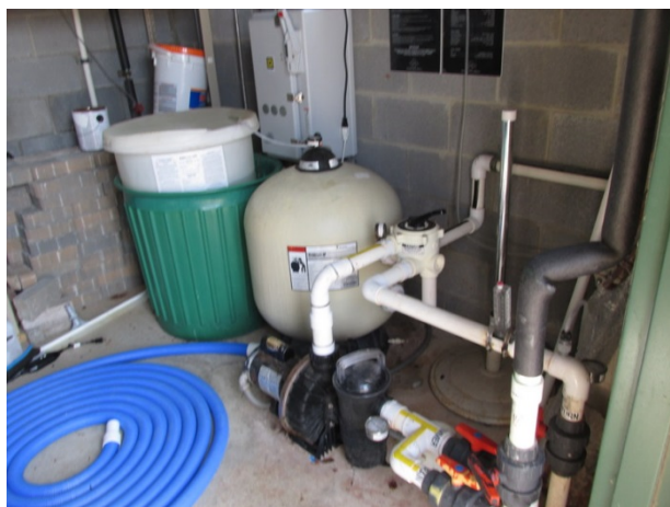
Wading pool mechanical equipment
