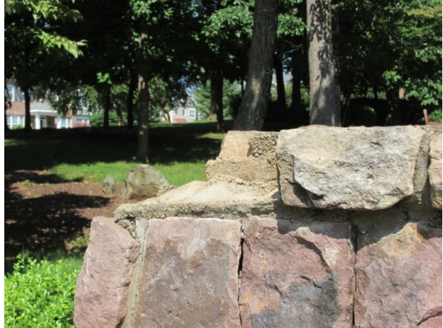
Missing masonry block
