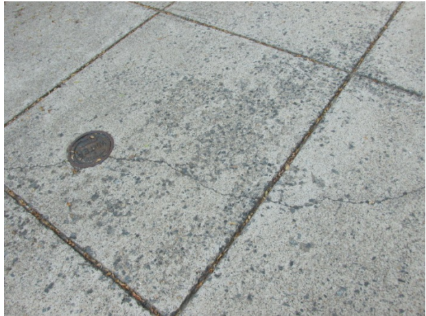
Concrete spall and cracks
