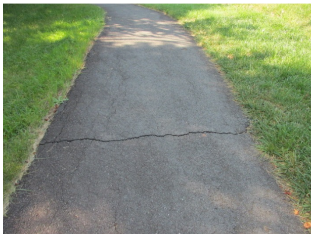
Walking path crack
