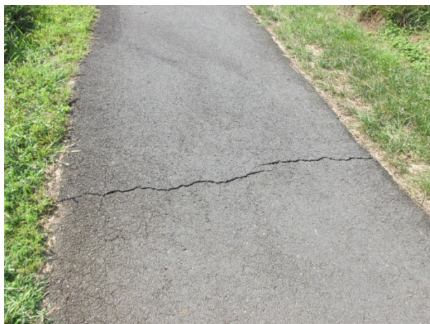
Walking path cracks
