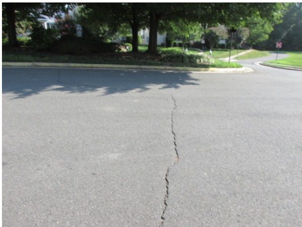
Pavement cracks at townhome pavement
