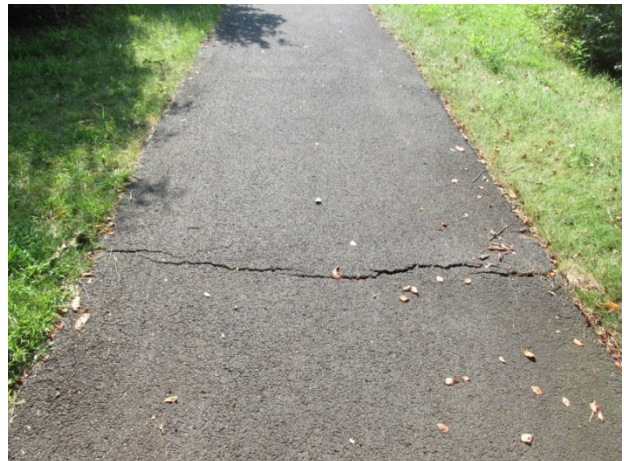
Walking path cracks
