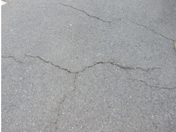
Pavement cracks at alley
