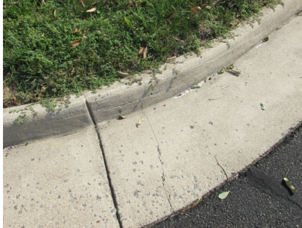
Curb and gutter crack
