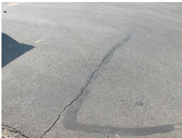
Cracks and previous repairs
