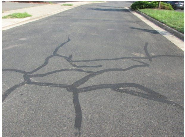
Previous repairs at townhome pavement
